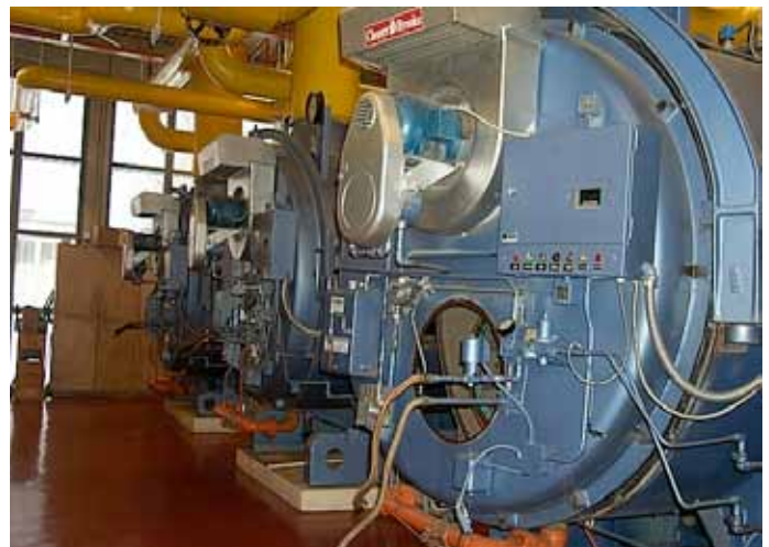
Boiler used for heating
